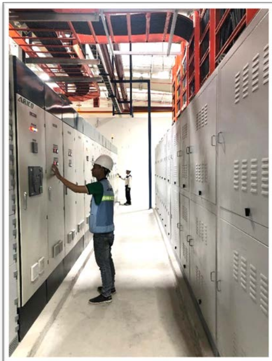
Start-up & Commissioning E.S
