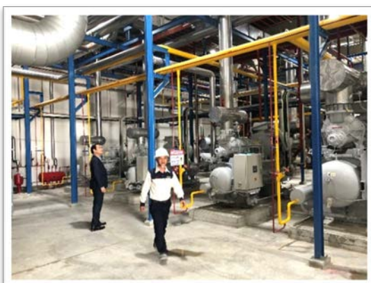
Inspection Refrigeration Machine Room
