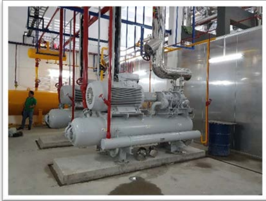
Chilled Water Thermal Storage System
