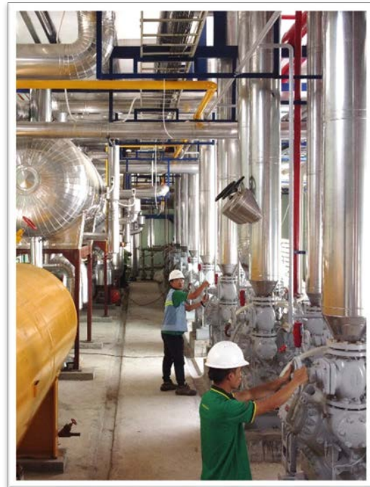
Start-up & Commissioning R.S
