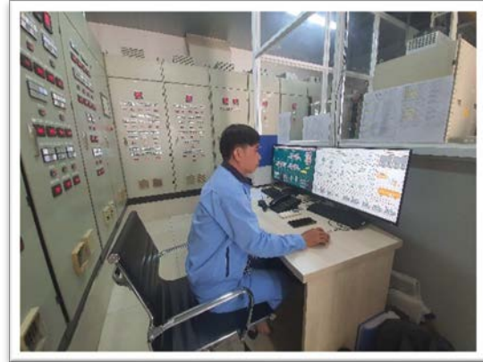
SCADA for Refrigeration System
